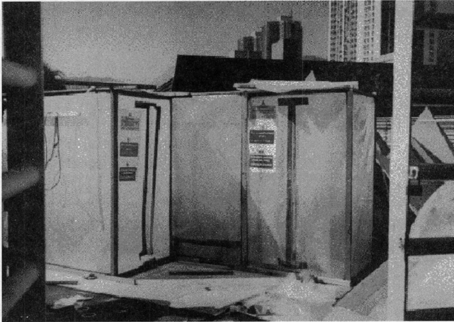
Plate 3 Decontamination Unit and Debris Port
