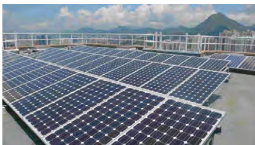
Mono-crystalline silicon PV panels installed at Lam Tin Estate Phases 7 & 8
