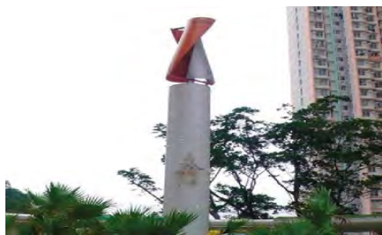
Wind-solar hybrid energy generating system for lighting at Sau Mau Ping South Estate
