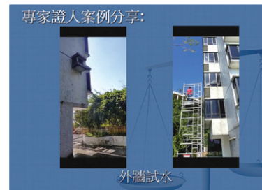
Figure 6: Tracing the Source of Water Penetration from an External Wall as an Expert Witness
